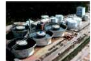
Waste Water Purification
