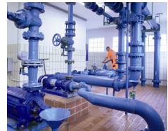
Water/Waste Water Complete solutions with controls, I/Os, infrastructure and wireless integration. Also, Networking of pump stations
